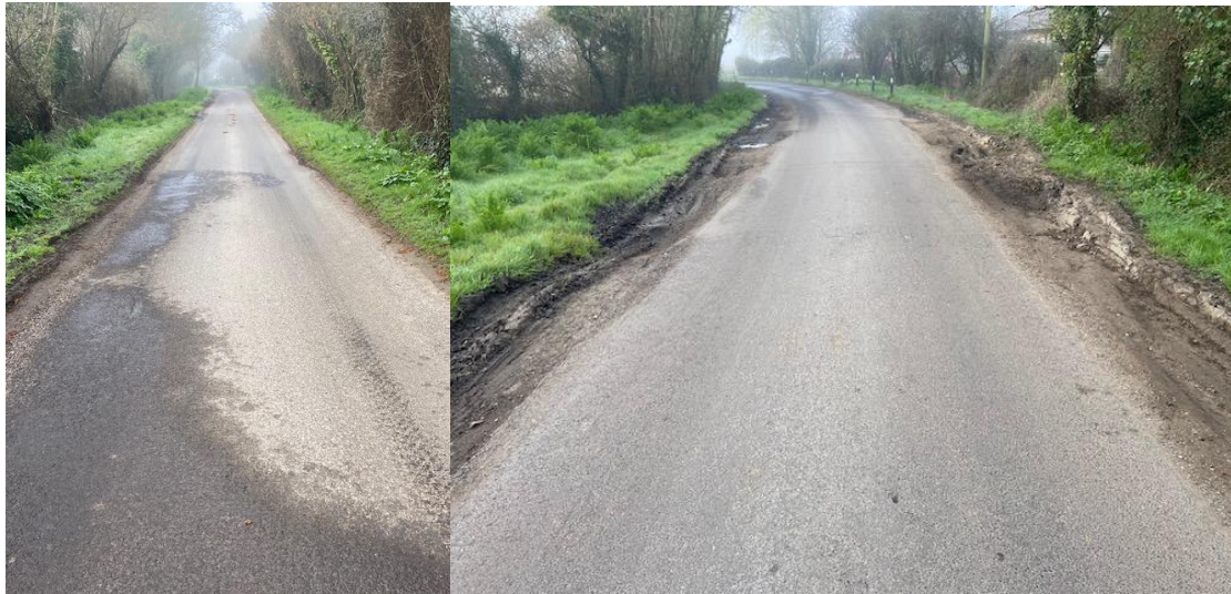
Road width 2.7m; badly damaged verges with deep, muddy potholes
