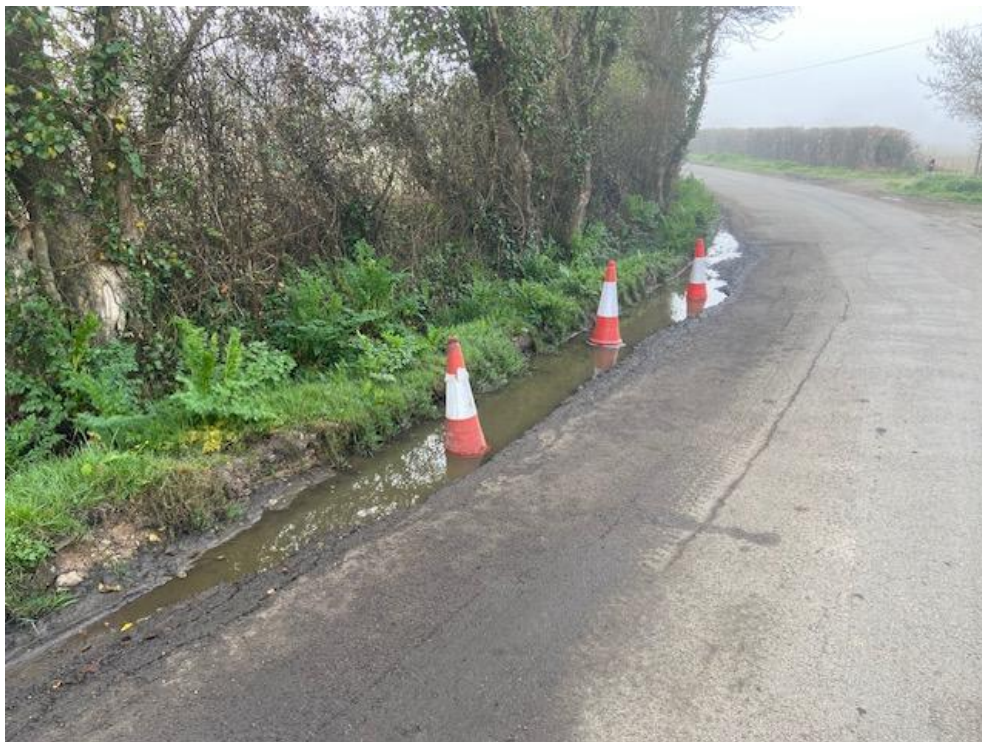
Large, deep trench on inside of bend 'hidden' by a long puddle
